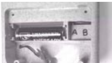
9V alkaline battery Back up power
