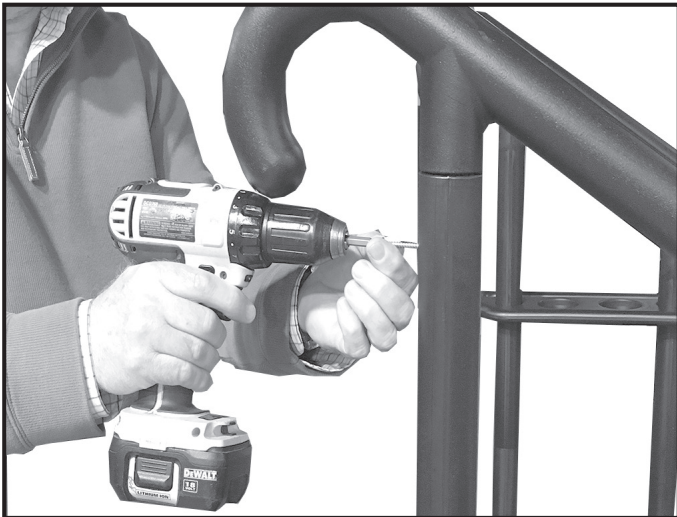
Step 9: Secure handrails using 1- #10 x 1¼" screw into each post at pre-marked locations.
